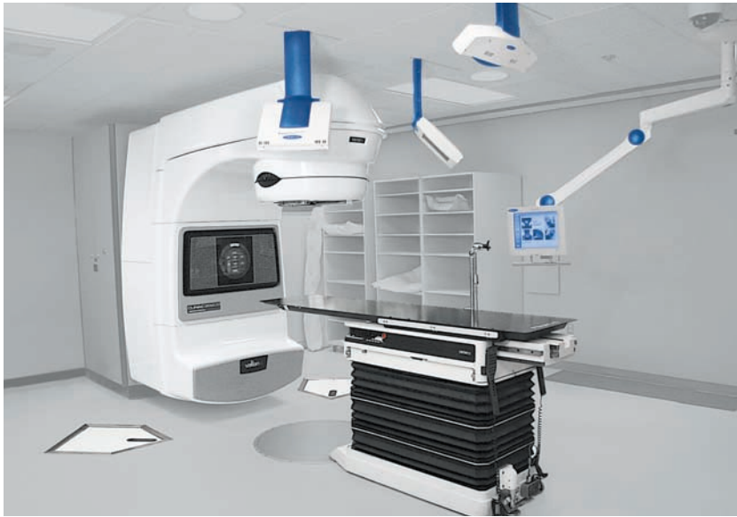
ExacTrac installed at CARTI, Little Rock, Arkansas, USA
